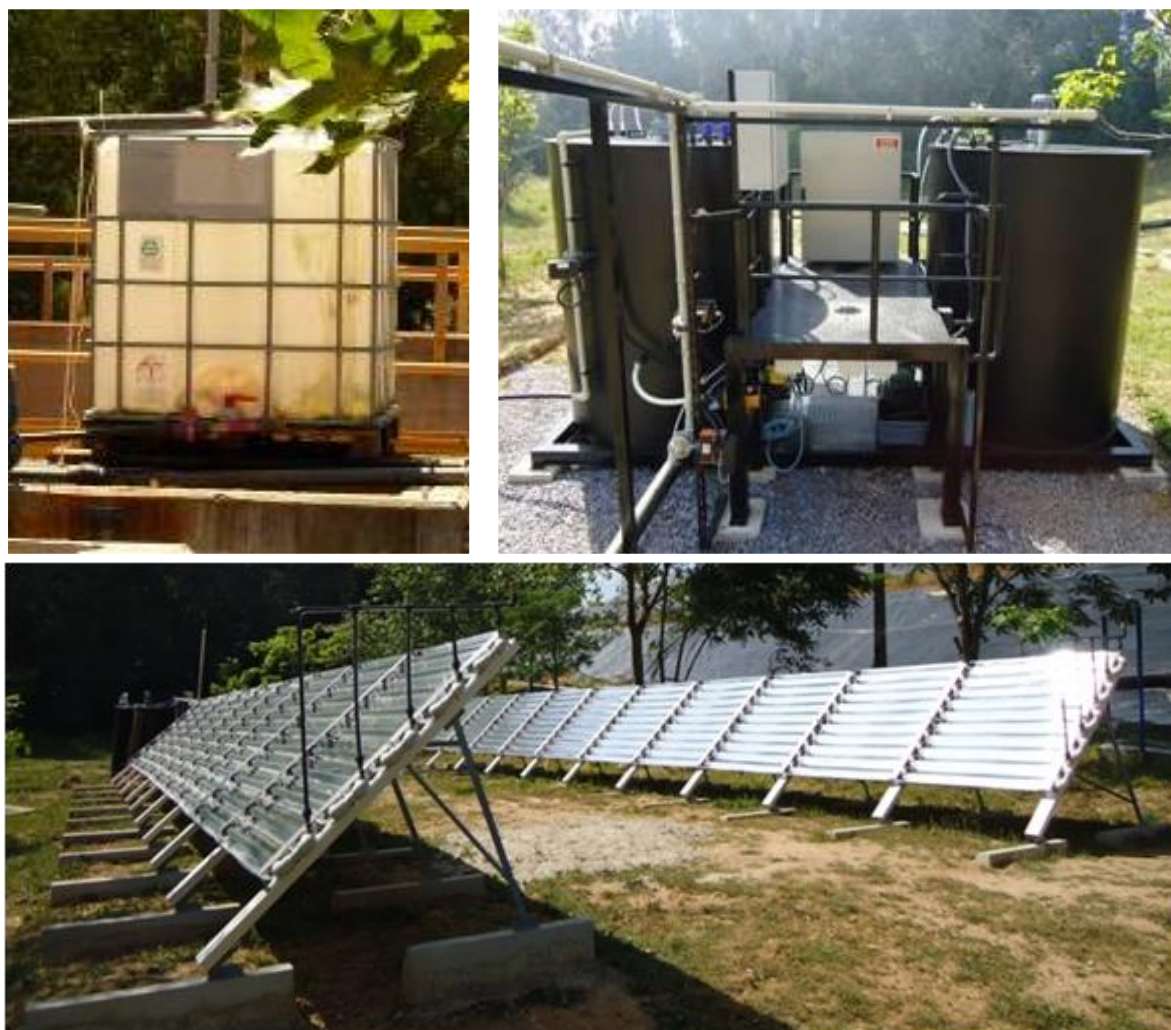
Figure 2.1. Solar pre-industrial unit combining photocatalytic and biological oxidation systems.
