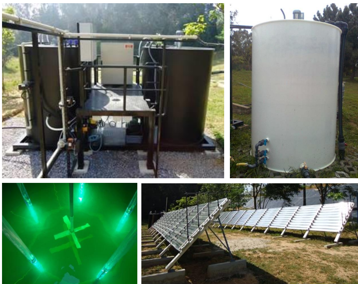
Figure 2.5. Solar/UV pre-industrial unit combining biological and chemical oxidation systems.
