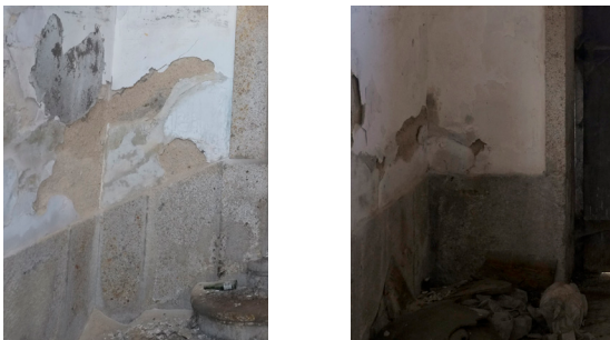
Figs.104 - 105 Danos no reboco
