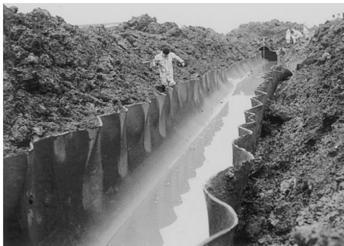
Figure 2.3 – Steel pipeline after long crack propagation (Makino et al., 2001).
