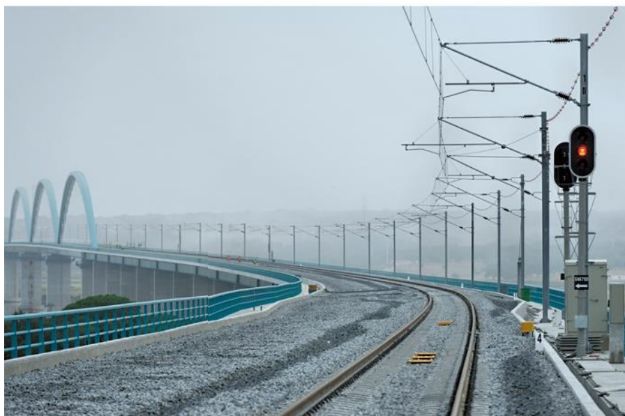
Figure 6.33 - Catenary and signalling system (REFER, 2010).
