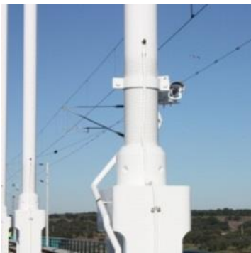
Figure 6.54 - IP camera installed in a hanger.
