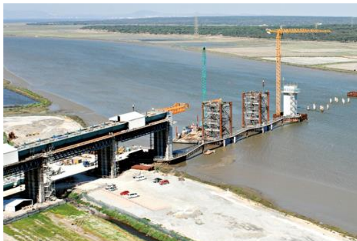
Figure 6.18 - Span of the bridge being assembled, over the South access viaduct (REFER, 2010).
