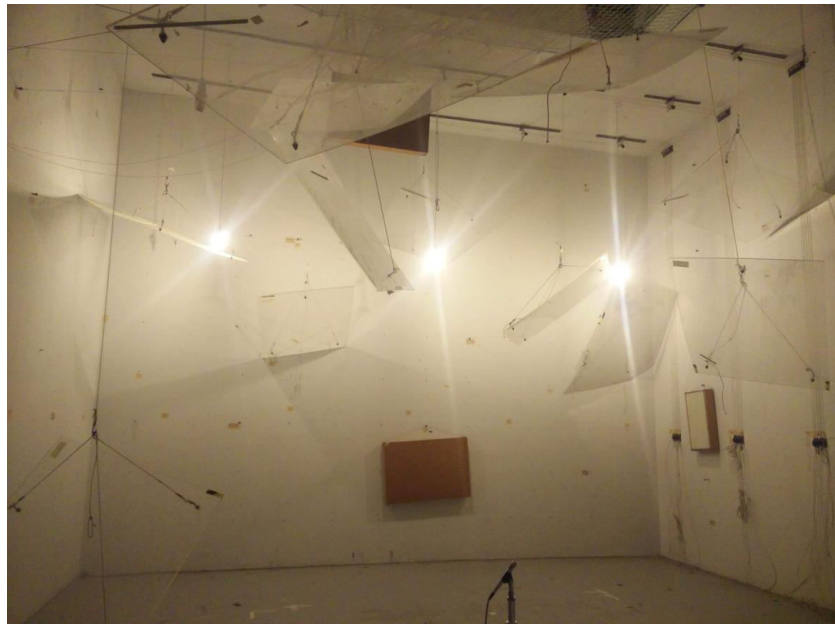
Figure 3.5: Panel diffusers in room 904
