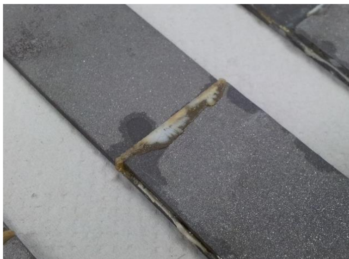
Figure 45. Burn marks encountered in the adhesive DP-8005 when 150°C temperature curing's were performed.
