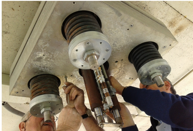
Fig. 1.5: Tuned Mass Damper instalado na ponte pedonal FEUP
