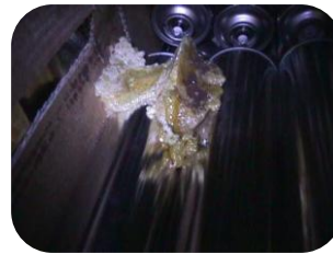
Example of foam released during the storage from a valve in bad state
