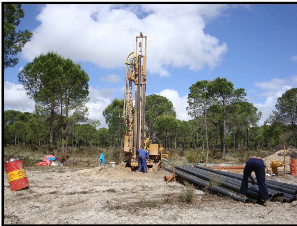
Fig. 12 – Pre-collar drill rig to drill over the tertiary sediments and steel casing to protect the drill hole from collapsing
