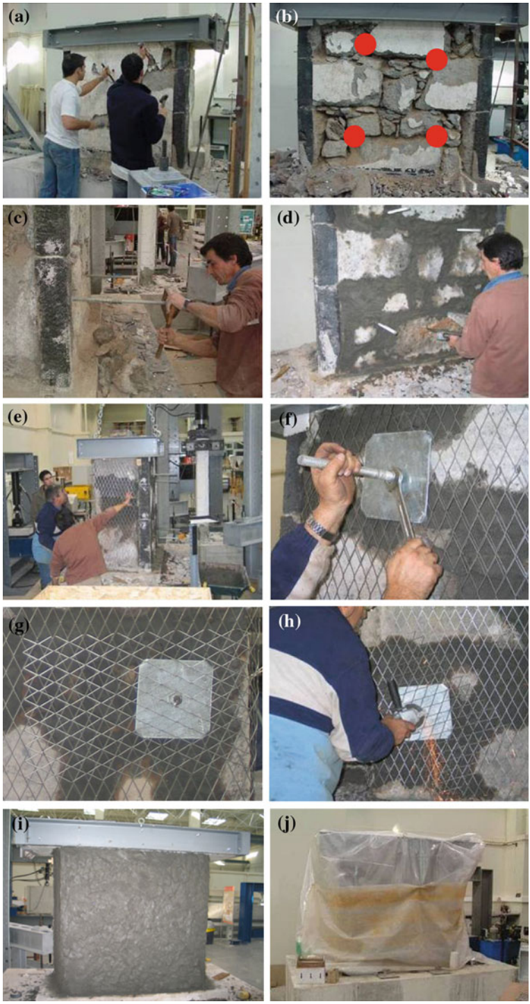
Fig. 22 Retrofitting technique used on the tested pier: from a–j as detailed in the text
