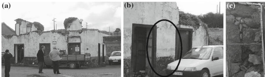
Fig. 2 Original location of the wall: a general view; b pier location; c wall cross-section
