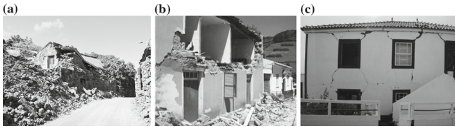
Fig. 1 Earthquake induced damages in Azores: a total collapse; b partial out-of-plane collapse; c in-plane damage
