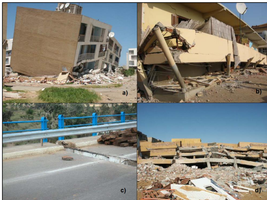
Figure 3.1 – a) Total displacement of the first floor; b) Elementary school in Corso, insufficient lateral resisting system; c) Damage to Highway 5 Bridge; d) Several floors pancaked (EERI, 2003)
