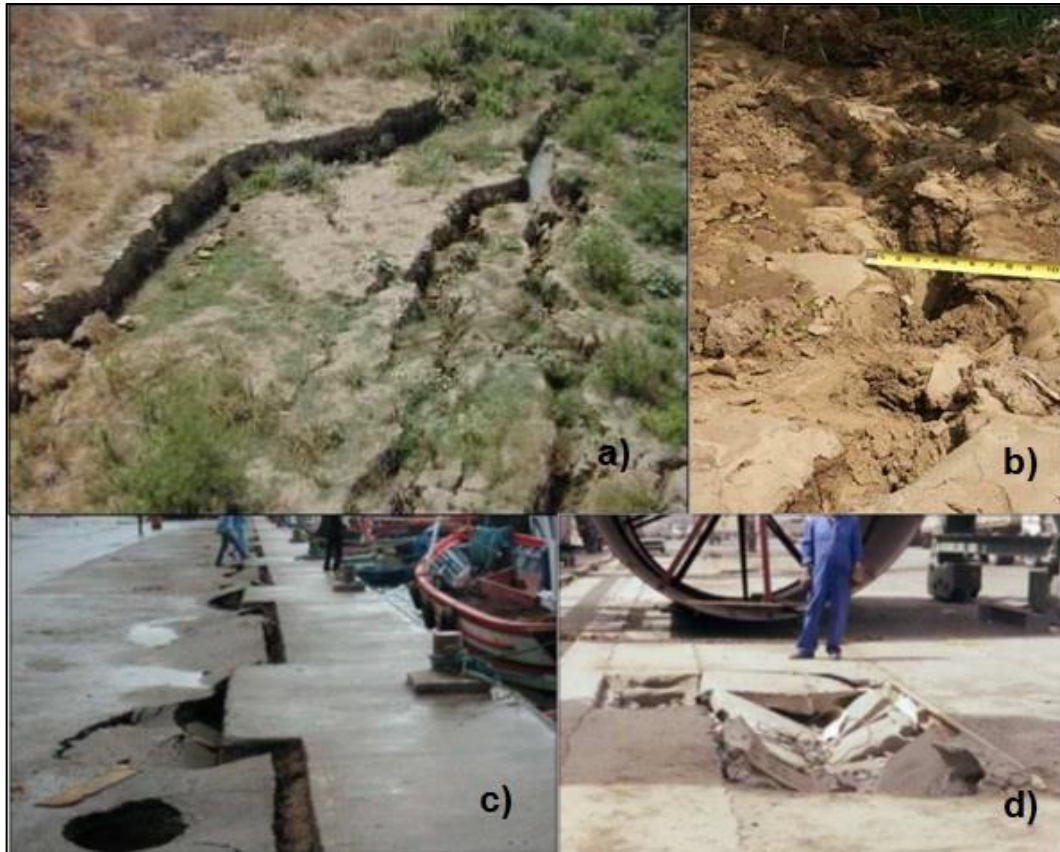
Figure 3.4 – a) Cracking; b) Sand boils ; c) and d) damage on roads due to liquefaction (EERI, 2003)
