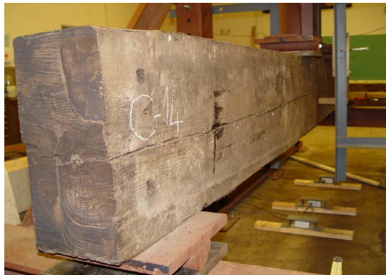
Figure 8: A horizontal shear crack [1].
