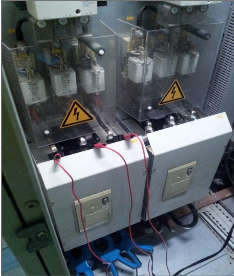
Figure 5.1 Picture taken during the audit, portraying the installation of a power quality analyzer
