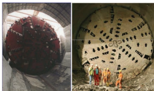
Fig. 2.3 – Tuneladora (Topa Gomes, 2010)
