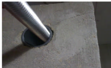
Figure 3.15 – Steel Bar in Contact with Concrete
