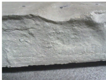
Figure 3.22 – Deformations on Concrete Frame
