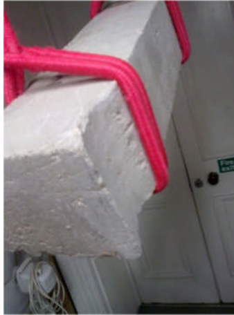
Figure 3.23 – Deformation on Concrete Frame
