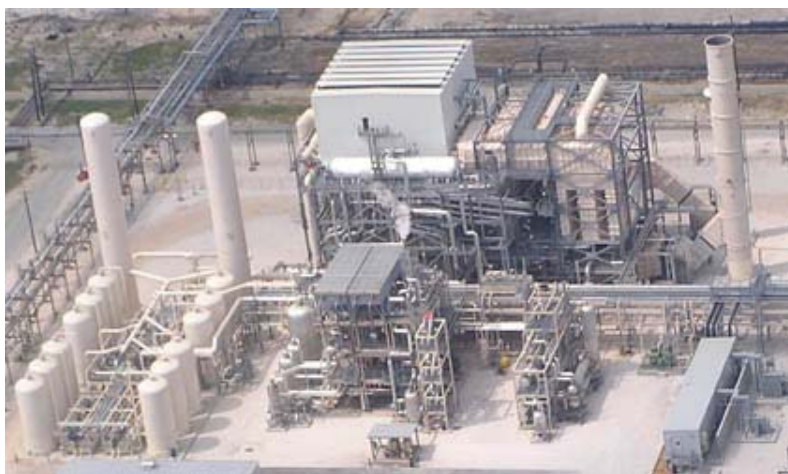
Figure 1.2. Methane steam reformer for the production of hydrogen ( \sim 112 \times 10^3 \text{ Nm}^3/\text{h} ) [9].
