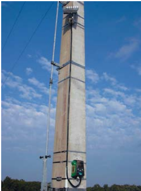
G200 unit with solar panel
