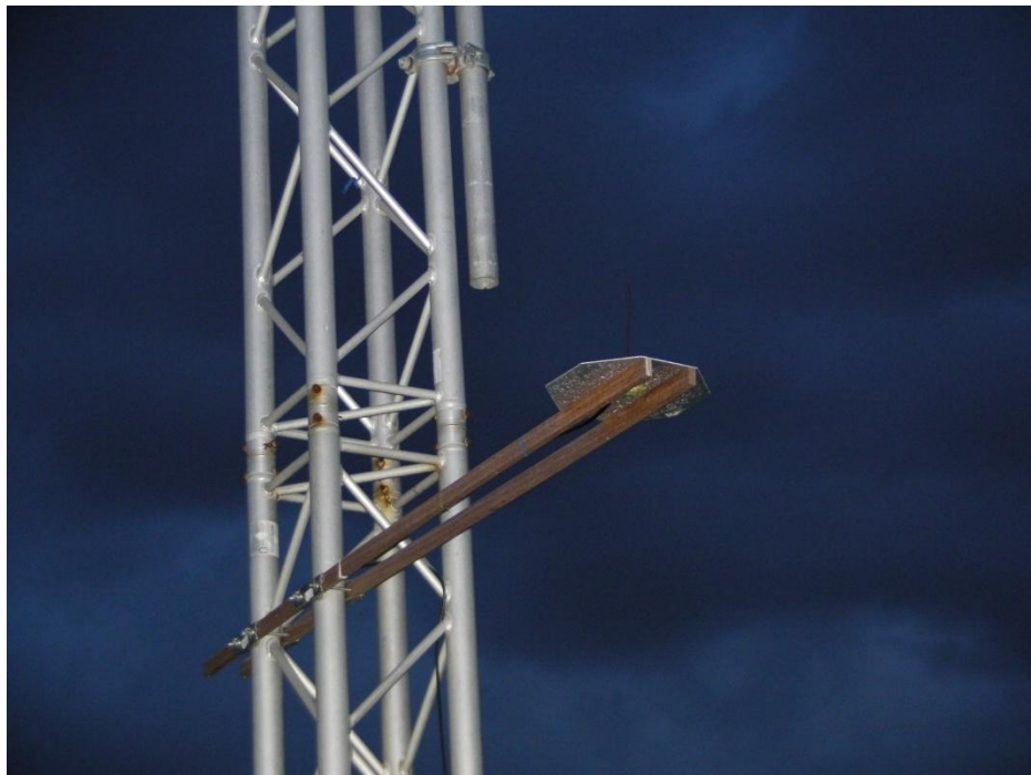
Figure 3.2 - Built antenna installed in the ground station roof.
