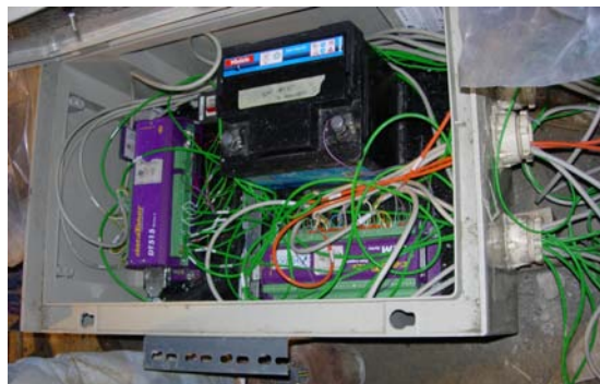
Figure 6.30: Datalogger system installed in the gallery
