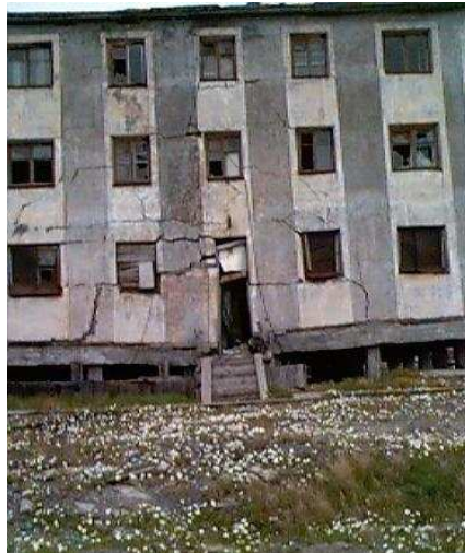
Fig.2.8 - Damage on a building provoked by the thawing of permafrost (Journal of Geocryology)
