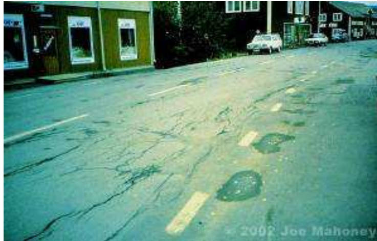
Fig.2.6 – Cracks on a pavement caused by frost heave (WAPA Asphalt Pavement Guide)
