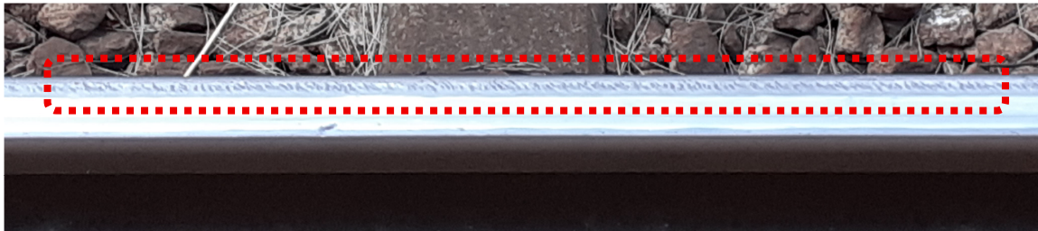
Figure 2.13: Picture of railway corrugation on the rail head, illustrating its periodic pattern that enables the use of frequency-based methods to detect this type of track defect.
