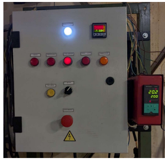
Figure 3.18: Electrical board: ASU2 burner malfunctioning light
