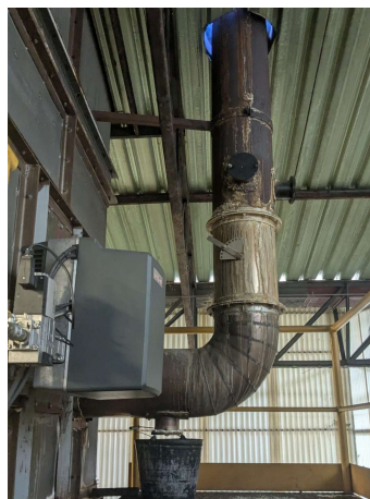
Figure 3.16: Acidic corrosion on the burner chimney
