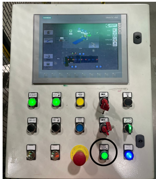
Figure 37: Modification made to the pre-feeder control system.
