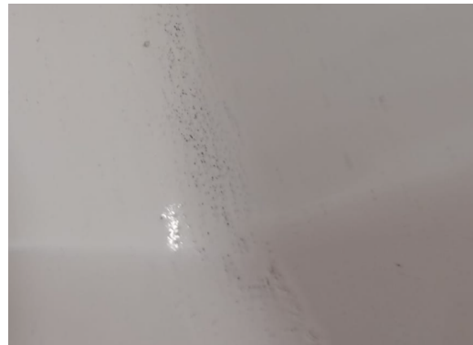
(b) Close-up of the defect.
