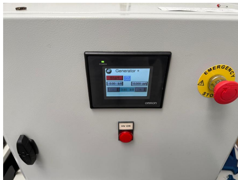
Figure 18 High-voltage generator (voltage source).
