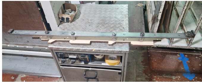
Figure 13: Second metal bar enabling external preparation of the blanking plate for the next order.
