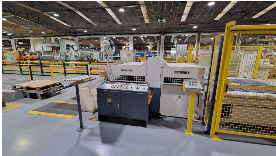
Figure 5: EasyBreak separator and palletising area.
