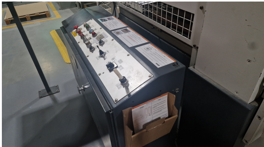
Figure 24: EasyBreak operating instructions installed at the machine.
