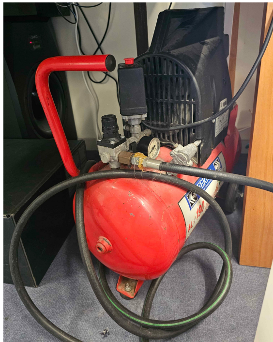
Figure 3.4: Air compressor sitting under the table
