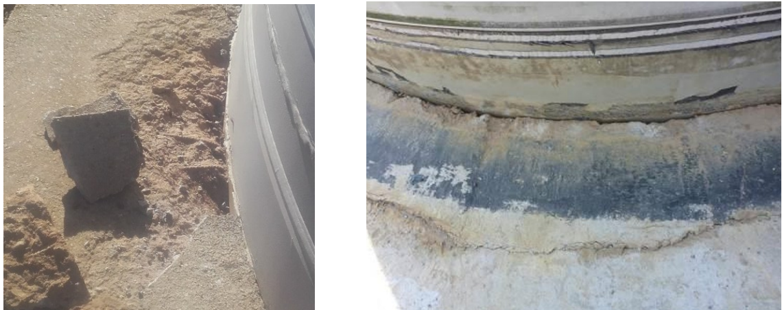
Figure 5.1 – Concrete spalling at the interface between the steel tower and concrete pedestal (photo on the right is courtesy from Kay Bode)
