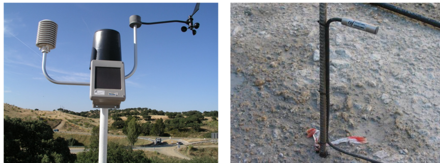
Figure 2.6: Weather station, including thermometers for air temperature measurement (left). Electrical resistance thermometer to be embedded in the dam body during its construction (right).
