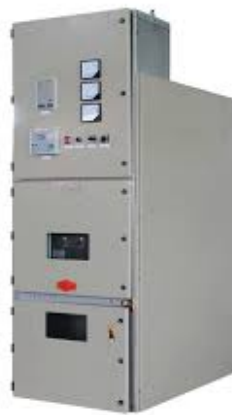
Figure 3.2: Medium Voltage Circuit Breaker
