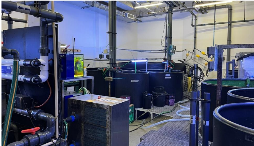
Figure 24 - Overview of SEA LIFE Porto's quarantine facility (Author: Maria Castelo).
