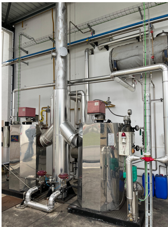
Figure 6.1: Current boilers in Socori 2
