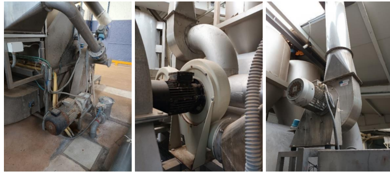
Figure 6.6: Motors Present in the Washing Process
