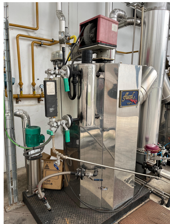
Figure 6.2: Detailed image of the boiler
