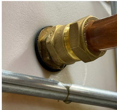
Figure 6.2: Example of leakage on a rubber sealant applied on a connection of the water tank.
