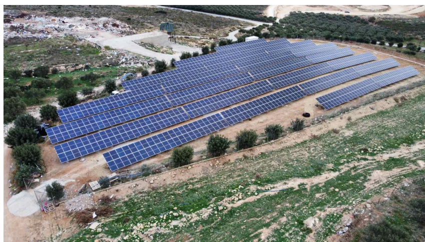
Figure 2.15: PV installation to supply REC in Minoia, Greece [63].
