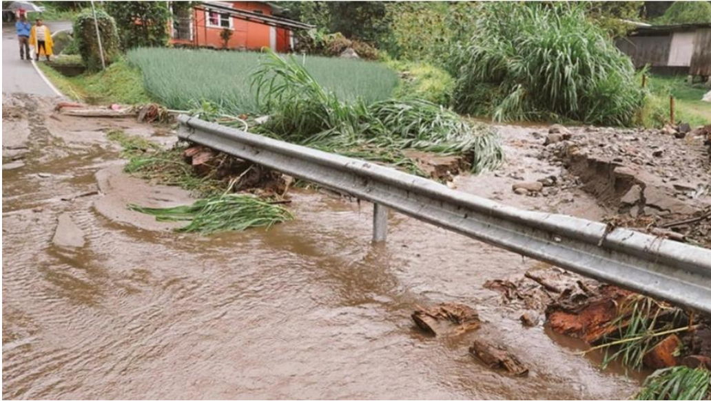
Fig. 34 - Flooding of the stream “La Chacha” in the Tierras Altas district due to heavy rainfall in the region [84].
