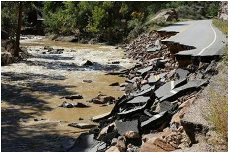
Fig. 1 - Colorado, USA; flooding damage [16].
