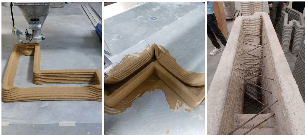
Figure 74 – Wall collapse of 3D-printed earth at the eighth layer of printing at long wall spans (left and center) (Courtesy: EcoMIT Project); Intermediate connectors (right) (Courtesy: Havelar).
