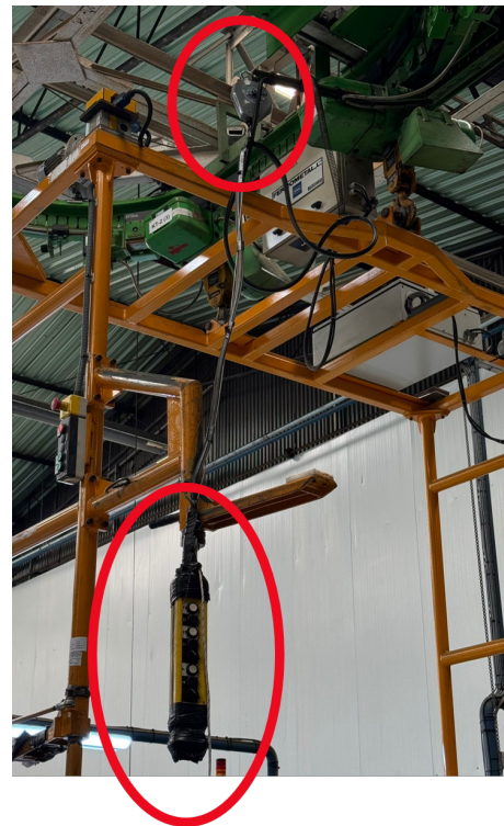
Figure C.19: Spring Balancer System installed
