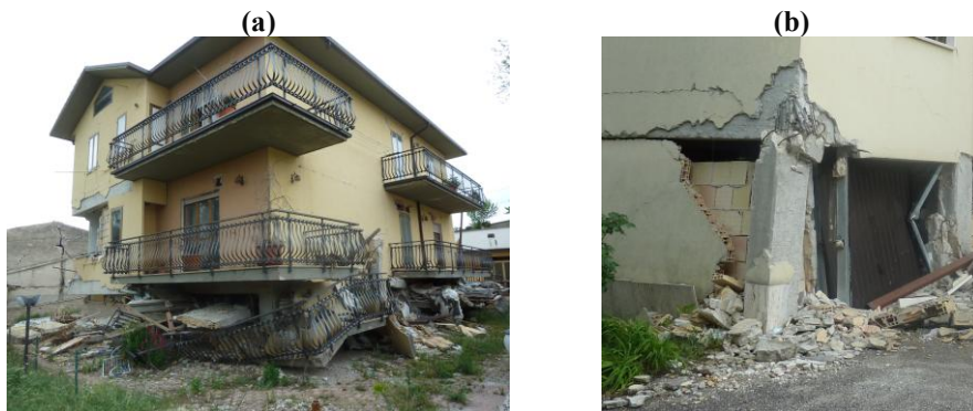
Figure 2-2: L'Aquila, Italy—2009: (a) damages on RC structure in L'Aquila; (b) node damage of reinforced concrete elements
