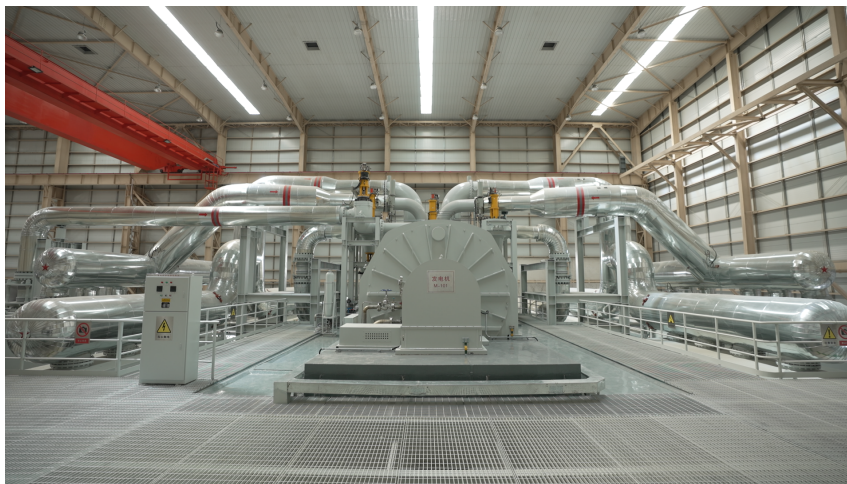
Figure 3.3: 100MW Compressed Air Energy Storage (CAES) in Zhangjiakou, Hebei Province, China, image by IET [34]
