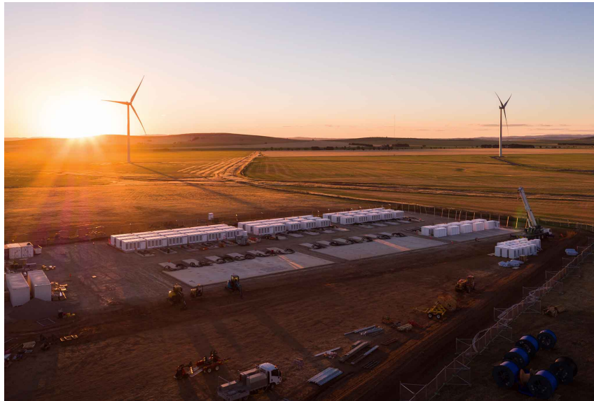
Figure 3.2: 150MW Lithium Battery Hornsdale Power Reserve, Australia [31] [32]
