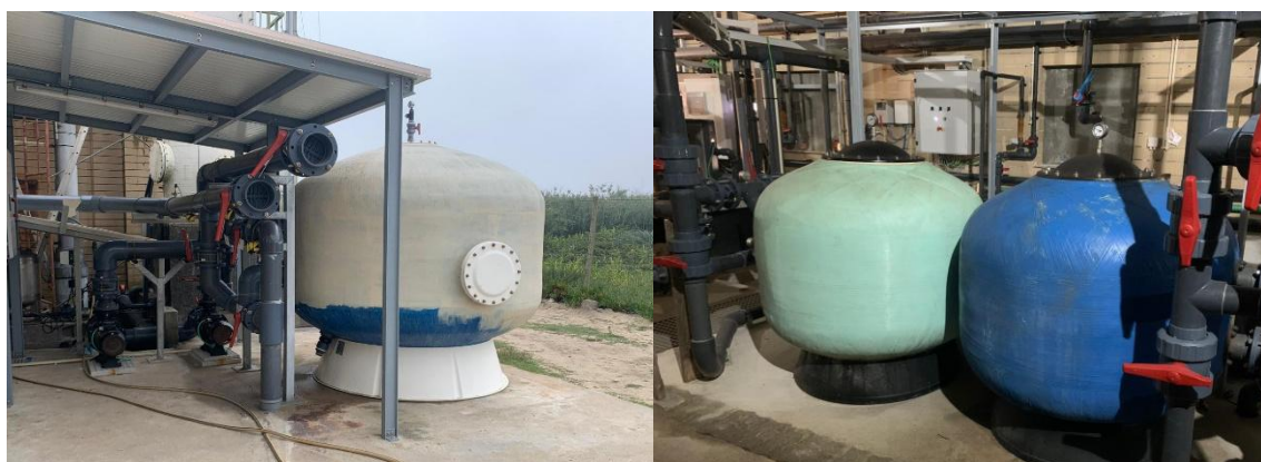
Figure 17 - Sand filters used in Safiestela. Photos taken by Alexandre Veloso.
