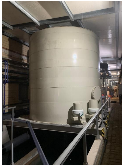
Figure 22 - Degassing tower used in Safietela. Photo taken by Alexandre Veloso.
