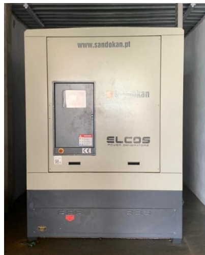
Figure 15 - Backup generator operated in Safiestela. Photo taken by Alexandre Veloso
