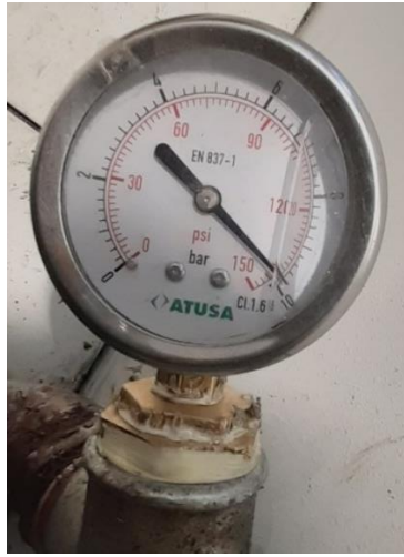
Figure 32- Gauge pressure at pump outlet.
