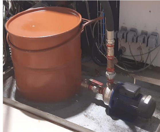
Figure 24- Small tank and return pump.
