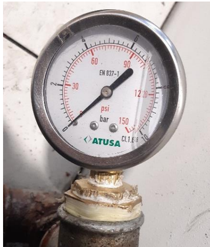
Figure 29- Pressure gauge installed on the pipes.
