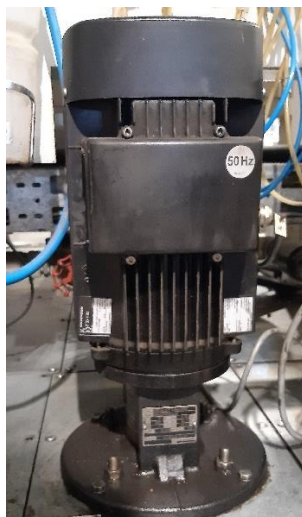
Figure 21- Installed pump above the tank.
