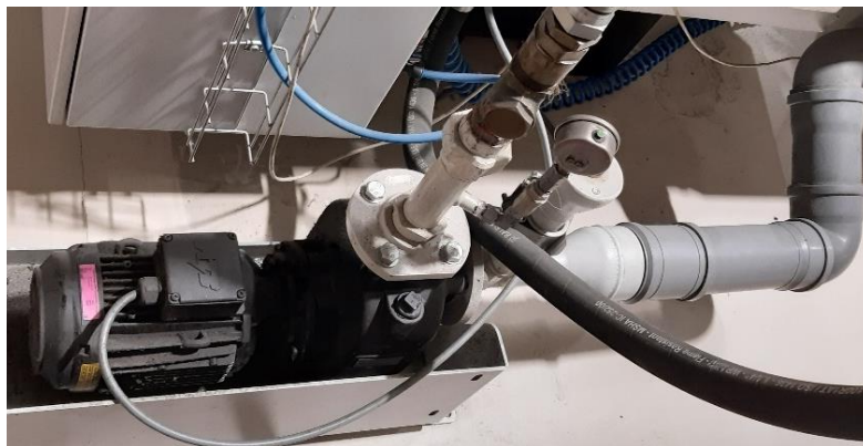
Figure 36- Return pump without auxiliary tank.
