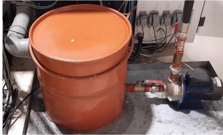
Figure 35- Small tank and pump to return the oil to the reservoir.
