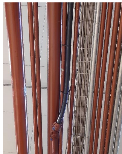
Figure 22- Pipelines where the oil circulates.
