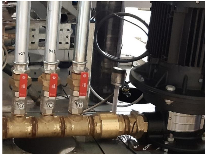
Figure 38- Manifold distributing oil through three different paths.
