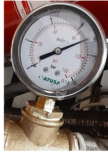
Figure 33- Pressure gauge at the machine inlet.
