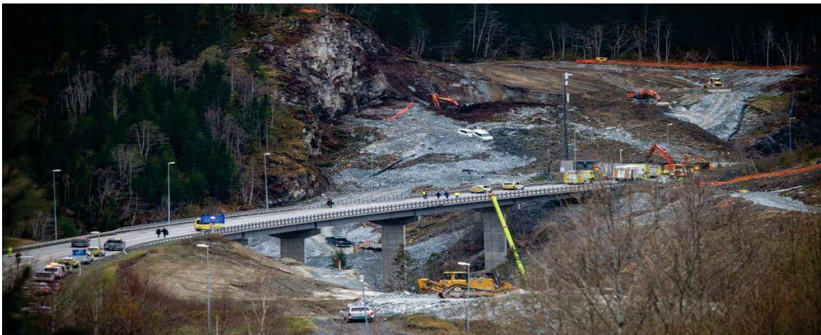
Figure 63 Landslide on the E6 highway in Norway[171]
