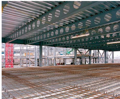
Figure 24 - Steel decking and cellular beams that are composite; Source (SCI, n.d.)
