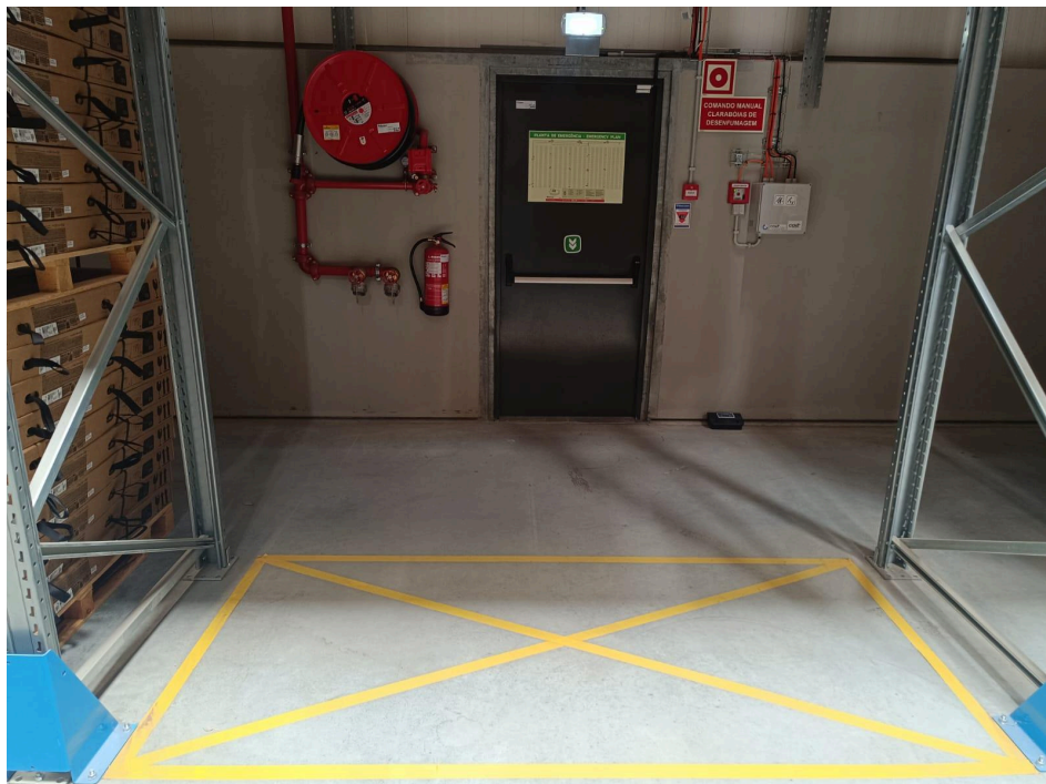
Figure 40 - Yellow Tape Markings for identifying an emergency exit
