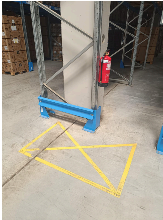
Figure 39 - Yellow Tape Markings for identifying an area occupied by a fire extinguisher
