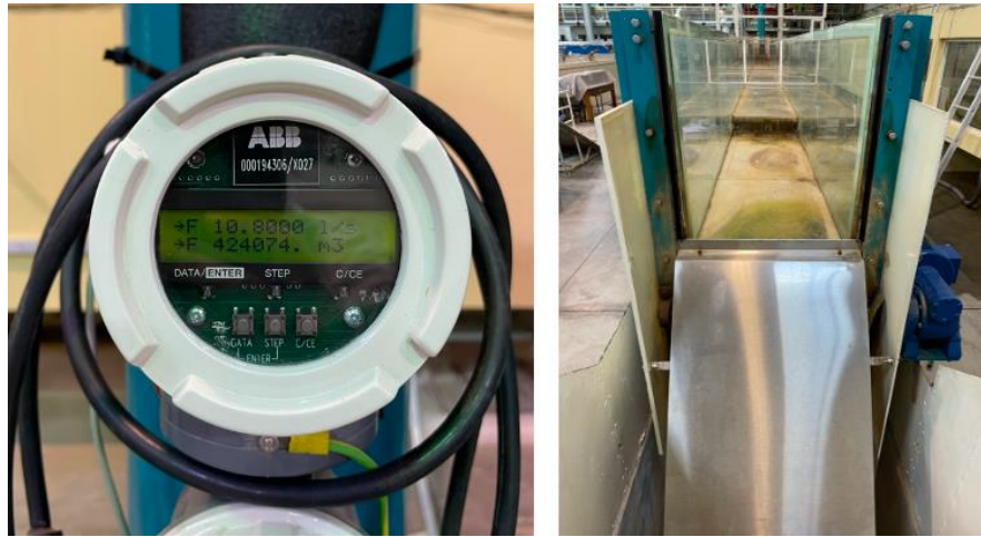
Figure 34. Flowmeter (Left); Electrical gate (Right)
