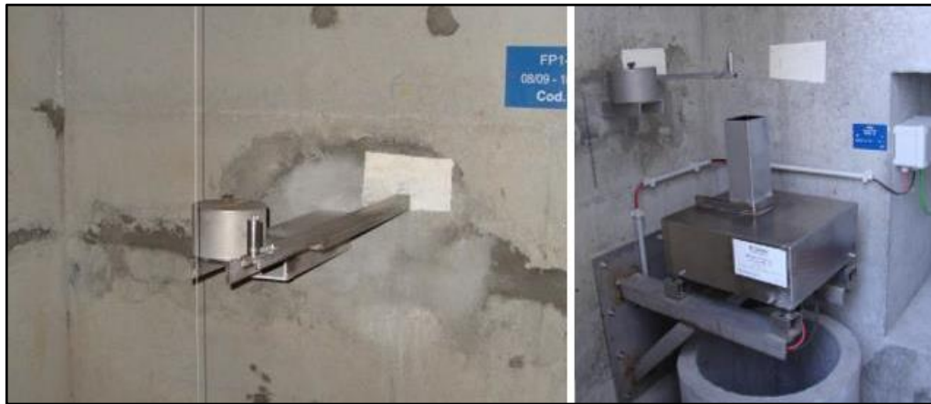
Fig. 6 - Plumb line and optical coordinometer (left) and tele-coordinometer (right), taken from (LNEC, 2020).
