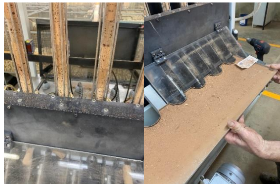
Figure 3.7: Examples of dust accumulation on CIP
