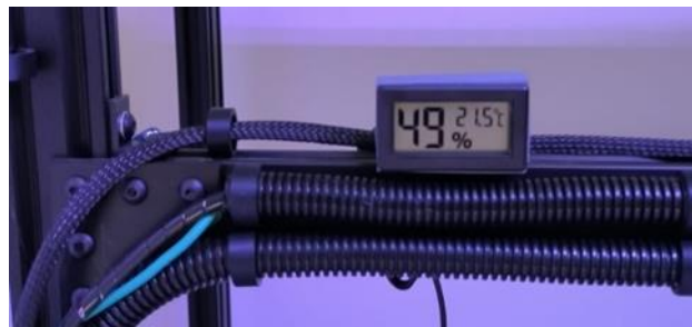
Figure 15 Temperature and Humidity control.
