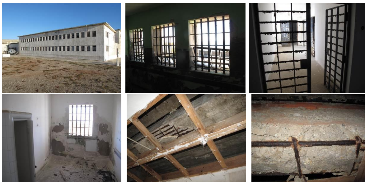
Fig. 20 – Former political prison buildings and their material/structural degradation
