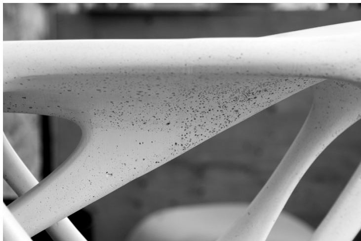
Figure 37. Close up of the air bubbles formed from the setting of the concrete.
