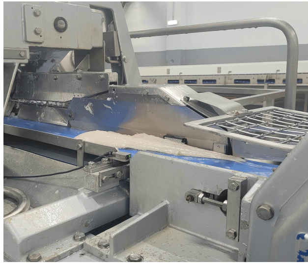
Figure 4.10: Omron E3ZM-R86 sensor installed
